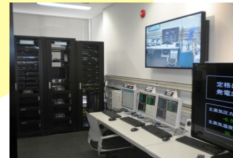
Thermal Electrical generating plant
