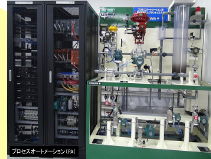
Sewerage and drainage process automation system
